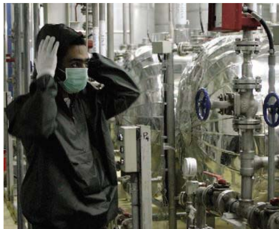
Condemnation. Iran resumed work at a uranium enrichment plant this month—an “unacceptable” action, according to the White House.
